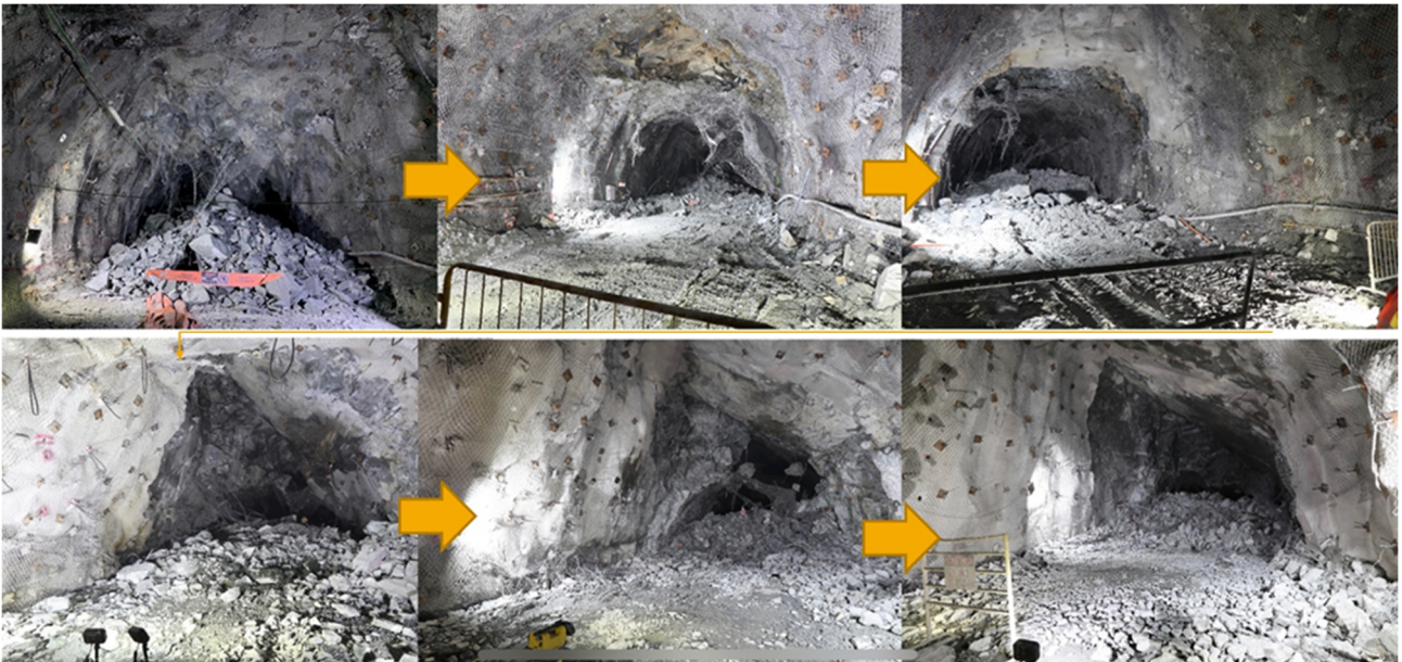
Figure 9 Rockburst rehabilitation process, including zones with deformed rock support system (Castro & Bahamondes 2020)
