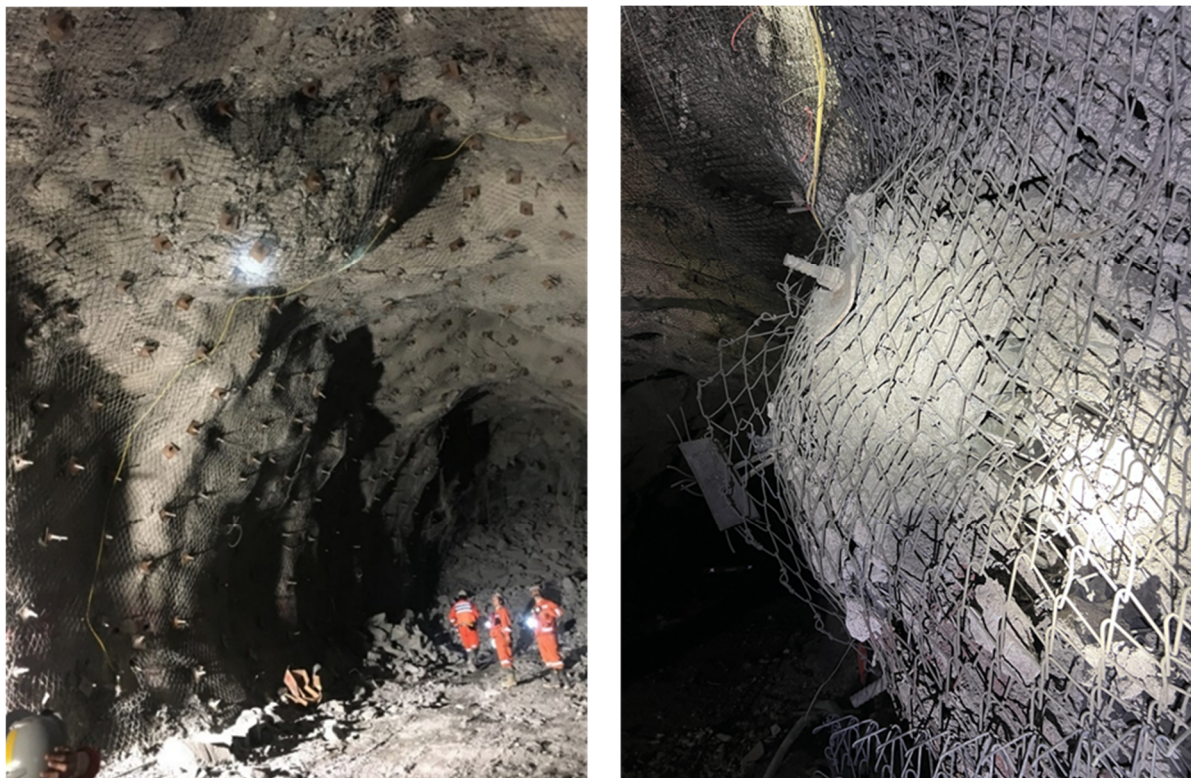
Figure 13 Photographic records with evidence of displacement of the rock mass contained by the support elements
