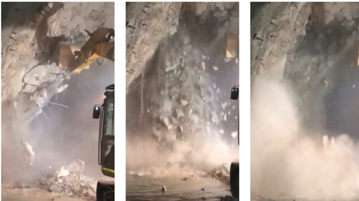
Figure 6 Rehabilitation process exposing rock fracturing behind retained volume by rock support system (operational ground control records)
