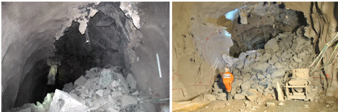
Figure 4 Rockburst damage after a seismic event M_w 2.0 in main infrastructure tunnels of the New Mine Level Project (Rojas et al. 2015)
